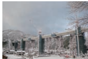
The new viaduct under construction in the snow. Upon completion, the concrete viaduct will measure approximately 310 meters long.
