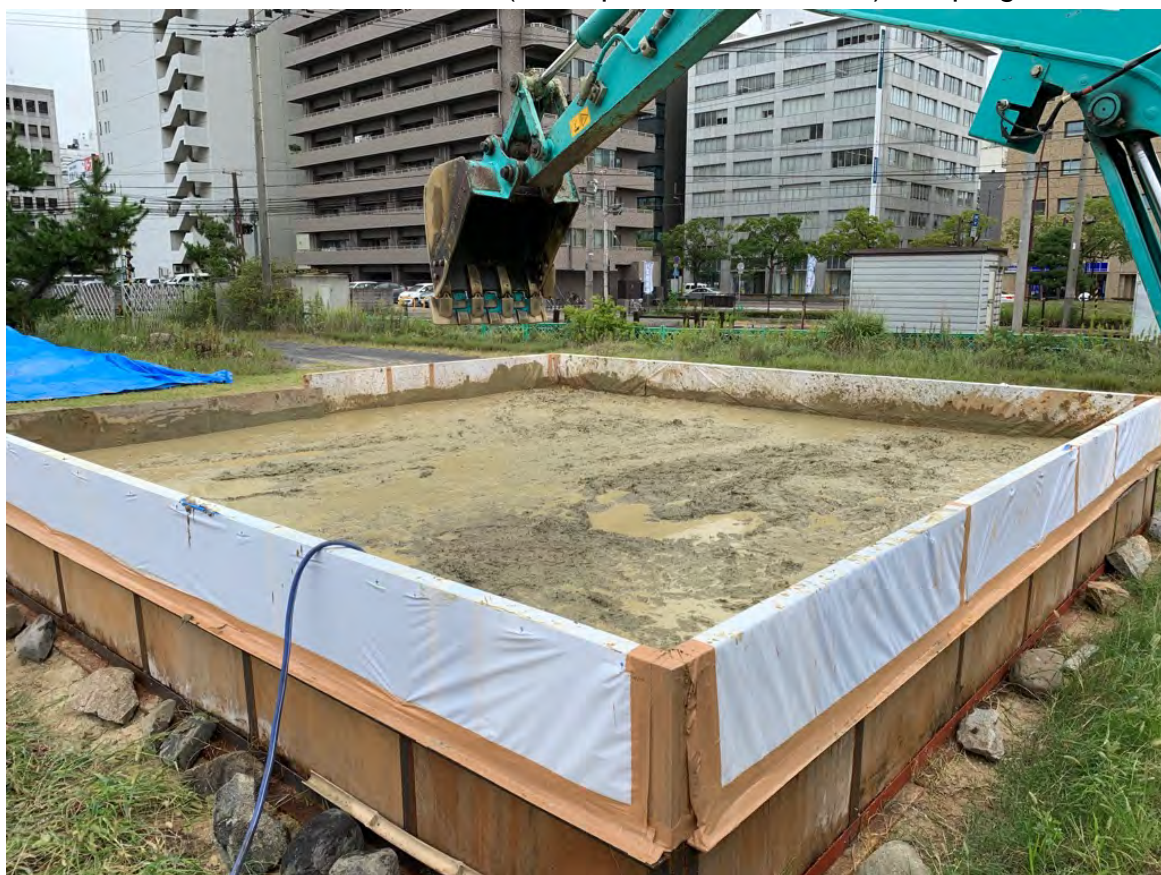
Mixing completed. After a further curing period, it will be mixed again.
