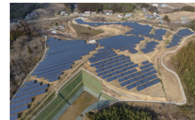
Solar power plant in Tome, Miyagi Prefecture
