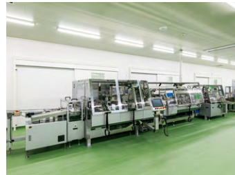
Packaging Line, Takaoka Plant, KYORIN Pharmaceutical Group Facilities Co., Ltd. (Takaoka City, Toyama Prefecture)
