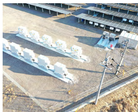
Kagoshima Isa Solar Power Plant and Energy Storage Facility (Isa City, Kagoshima Prefecture) Top: Solar Power Plant / Bottom: Battery Storage System
