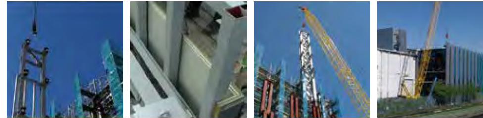
地組された組柱を仮置場に設置 Connected columns assembled at the site are placed in the temporary staging area 仮置場で組柱に外壁を取付 Outer wall is connected to connected columns in the temporary staging area 外壁と一体となった組柱の建方 Erection of integrated outer wall and connected columns 建方全景 Overall view of erection
