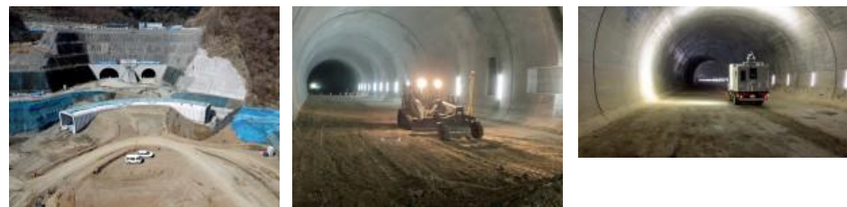
Japan Society of Civil Engineers Award, Ministry of Technology I (FY2022) Tunnel construction that realized productivity improvement by utilizing full ICT- (Shin-Tomei Expressway Kawanishi Construction Yagayama Tunnel)
