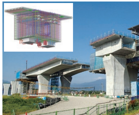
Using 3D modeling to check for clash between rebars and PC steel materials (Komaki Viaduct)
