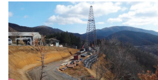
A geothermal power project (Oita Prefecture)
