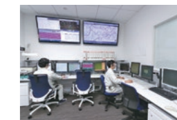
Shimizu's 24-hour building management center
