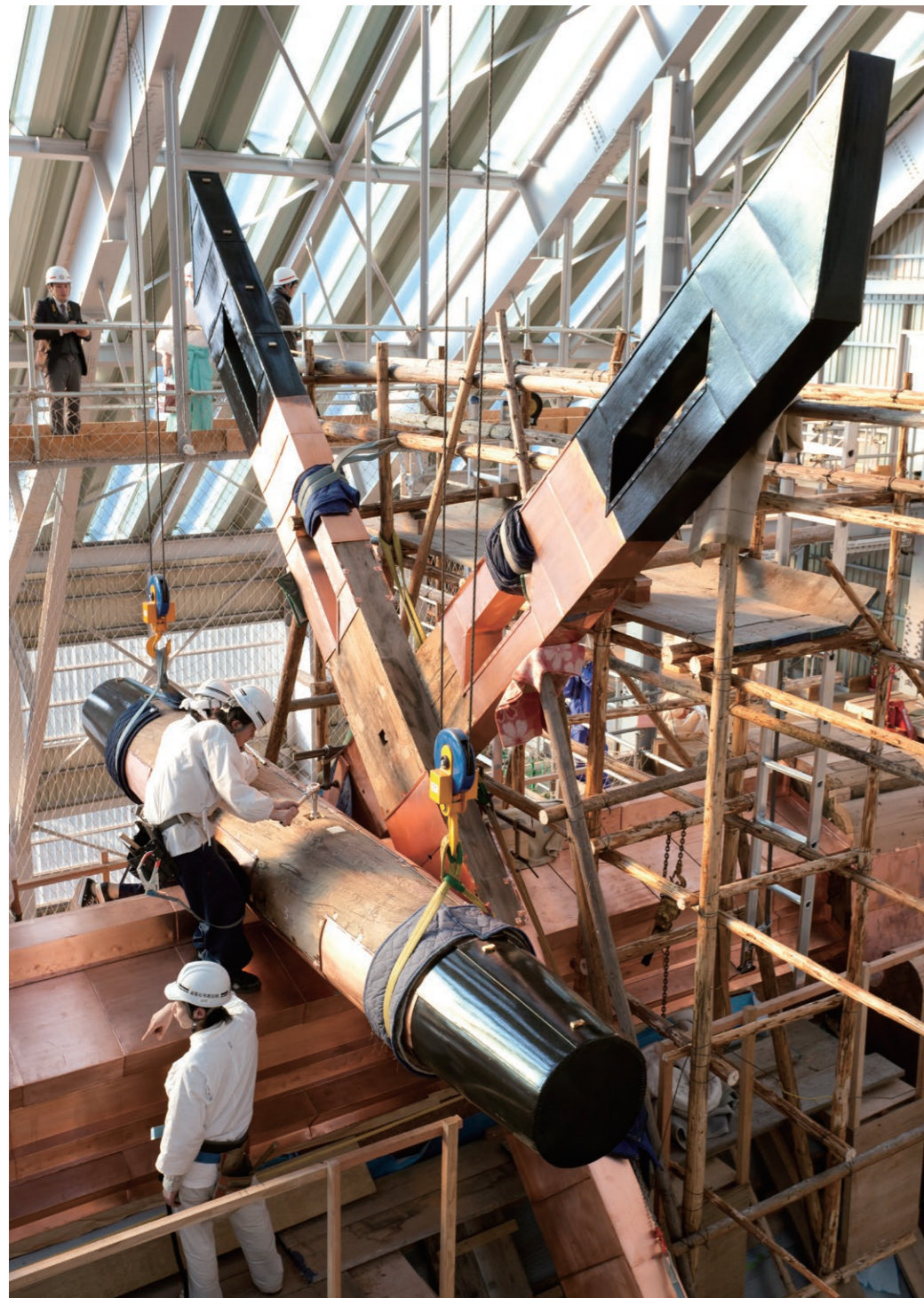
B Installing the restored log called katsuogi on the main shrine roof
