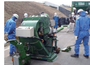
Work on the Ministry of the Environment's full-scale decontamination project in Okuma
