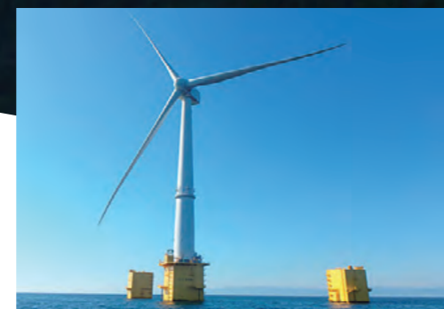
Fukushima Floating Offshore Wind Farm Demonstration Project (Photo: Fukushima Offshore Wind Consortium) This Fukushima Floating Offshore Wind Farm Demonstration Project (sponsored by the Ministry of Economy, Trade and Industry (METI)) is operating the world's first floating wind farm with multiple wind turbines off the coast of Fukushima Prefecture. Shimizu installed a 2 MW floating wind turbine in 2013 and 7 MW in 2015.
