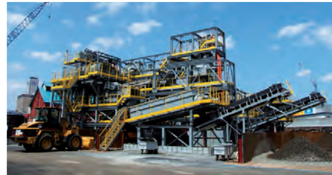
Dioxin washing plant
