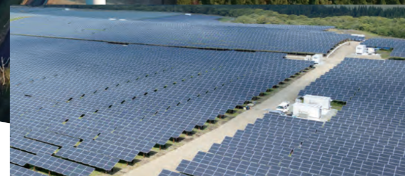
Eurus Rokkasho Solar Park Shimizu built the Eurus Rokkasho Solar Park, the largest mega solar project in Japan, in the village of Rokkasho in Kamikita-gun, Aomori Prefecture in 2015. It has a power generation capacity of 115,000 KW (enough electricity to power roughly 38,000 typical households), and contributes to reduction in CO 2 emissions of around 70,000 tons a year. Shimizu also operates the mega solar power plants it built in Ako, Hyogo Prefecture and in Kitakami, Iwate Prefecture.
