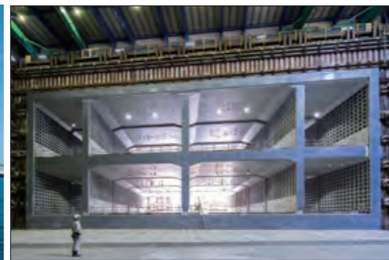
Construction of the Keisei Sugano Underpass on the Outer Ring Expressway — Jacked box construction directly beneath an operating railway line using the R&C construction method for a box with the largest cross-section in the world —
